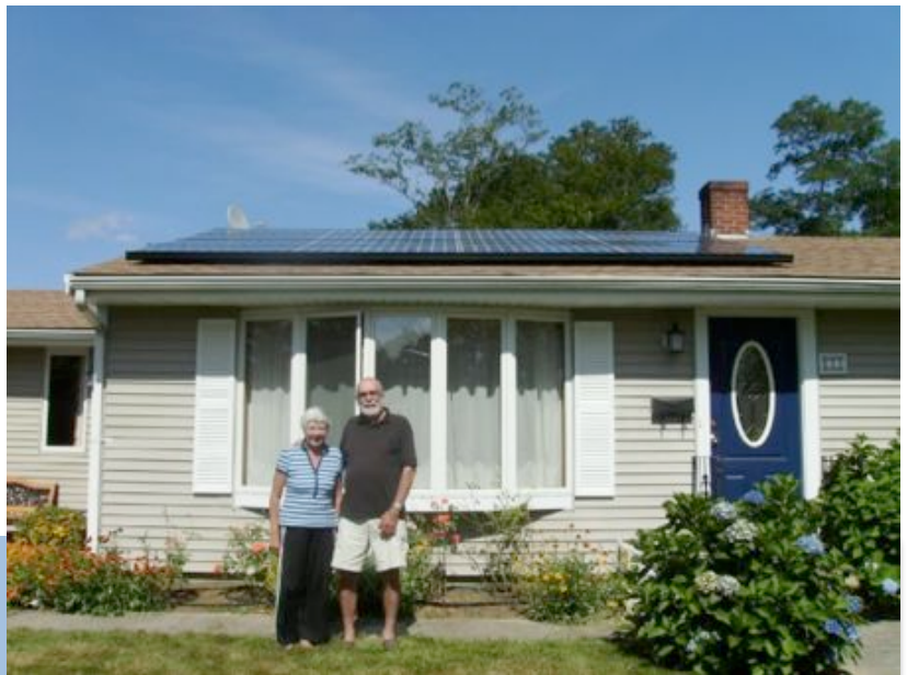
3.8kW Roof Mounted Solar Array
