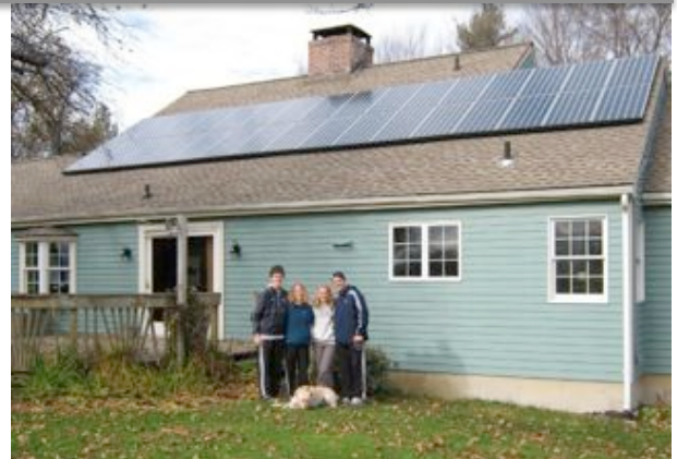
7.3kW Roof Mounted Solar Array
