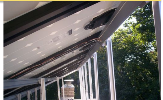
Back View of Tilted Panels
