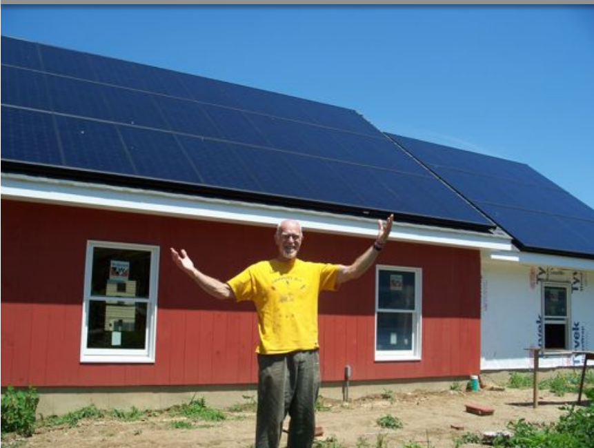
9.23kW Roof Mounted Solar Array
