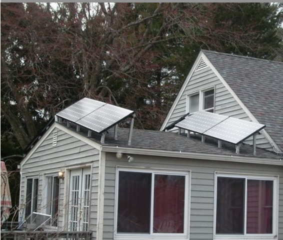
East Facing Roof with Southern Tilt Mounts
