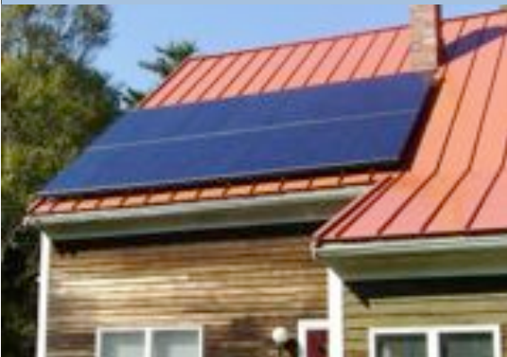
3.1kW Array Mounted on Metal Roof
