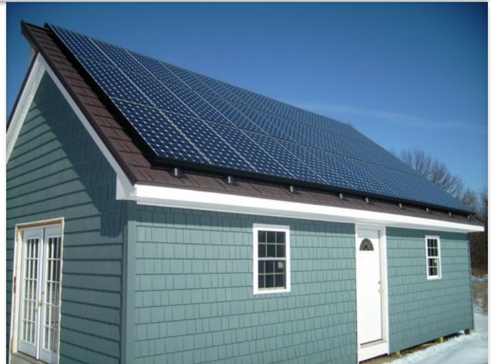
Part of an 18.63 kW Solar Array
