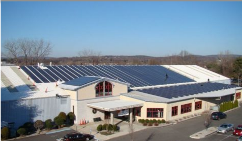
North Haven Health & Racquet Club, 190kW Solar Array
