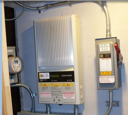
Inverter and DC Disconnect
