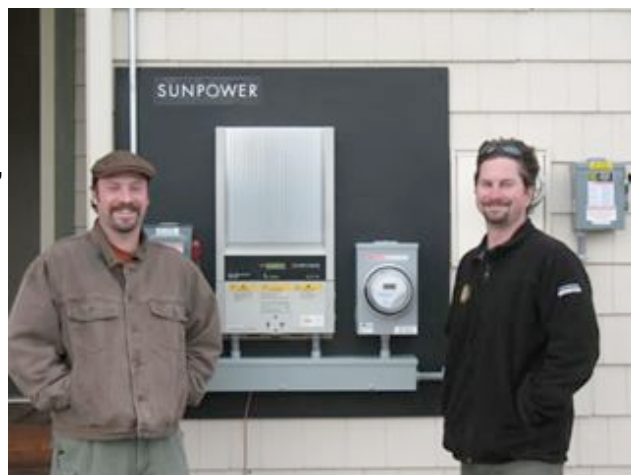
2.05kW PV Electrical Board
